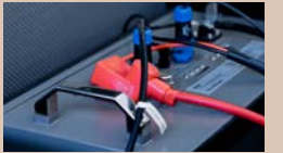
48 Voltage E175 Battery
